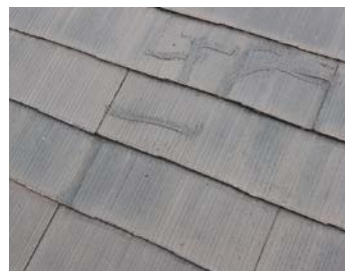
補修・塗装剥げ
